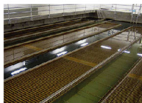
MAPLE GROVE DRINKING WTP
