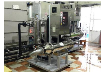
Seaweed Disinfection System
