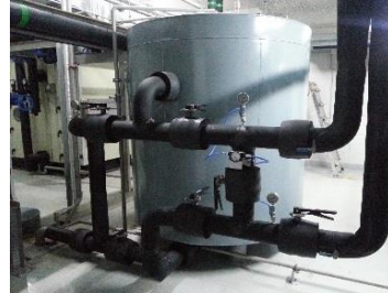
Arsenic removal System
