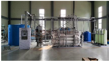
Malaysia Demi water treatment
