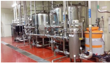
Haitai Beverage water treatment
