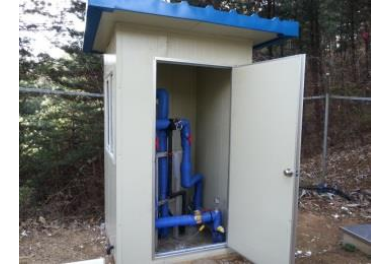
Gapyeong arsenic removal
