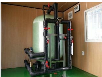
Hawcheon arsenic removal
