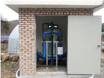
Samcheok-si arsenic removal
